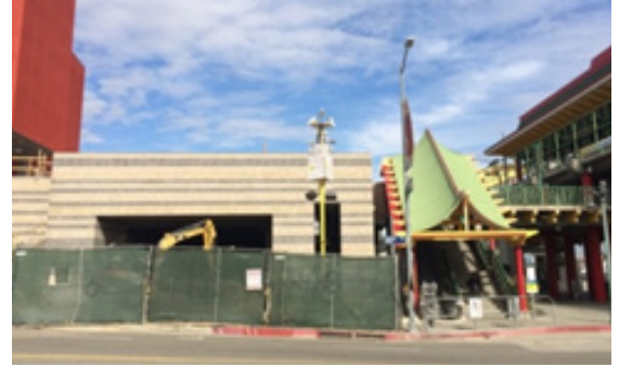
Sidewalk access is blocked for a construction project, forcing pedestrians into the street or to use less direct paths to the Metro facility.
